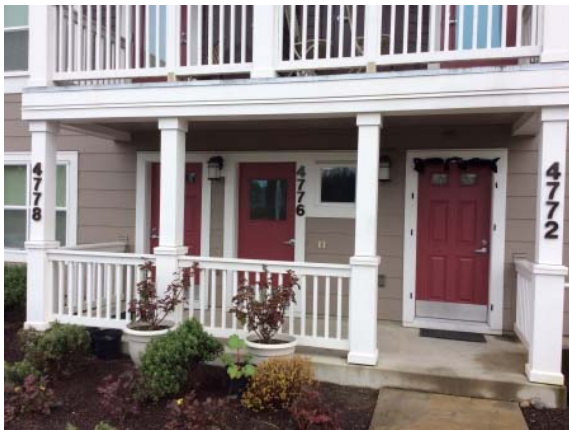
Photo #17: Apartment patio and balcony guardrail
