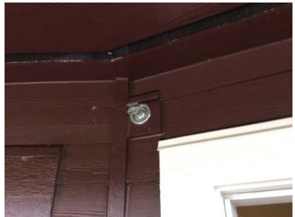
Photo #18: Soffit vent and exterior fire sprinkler
